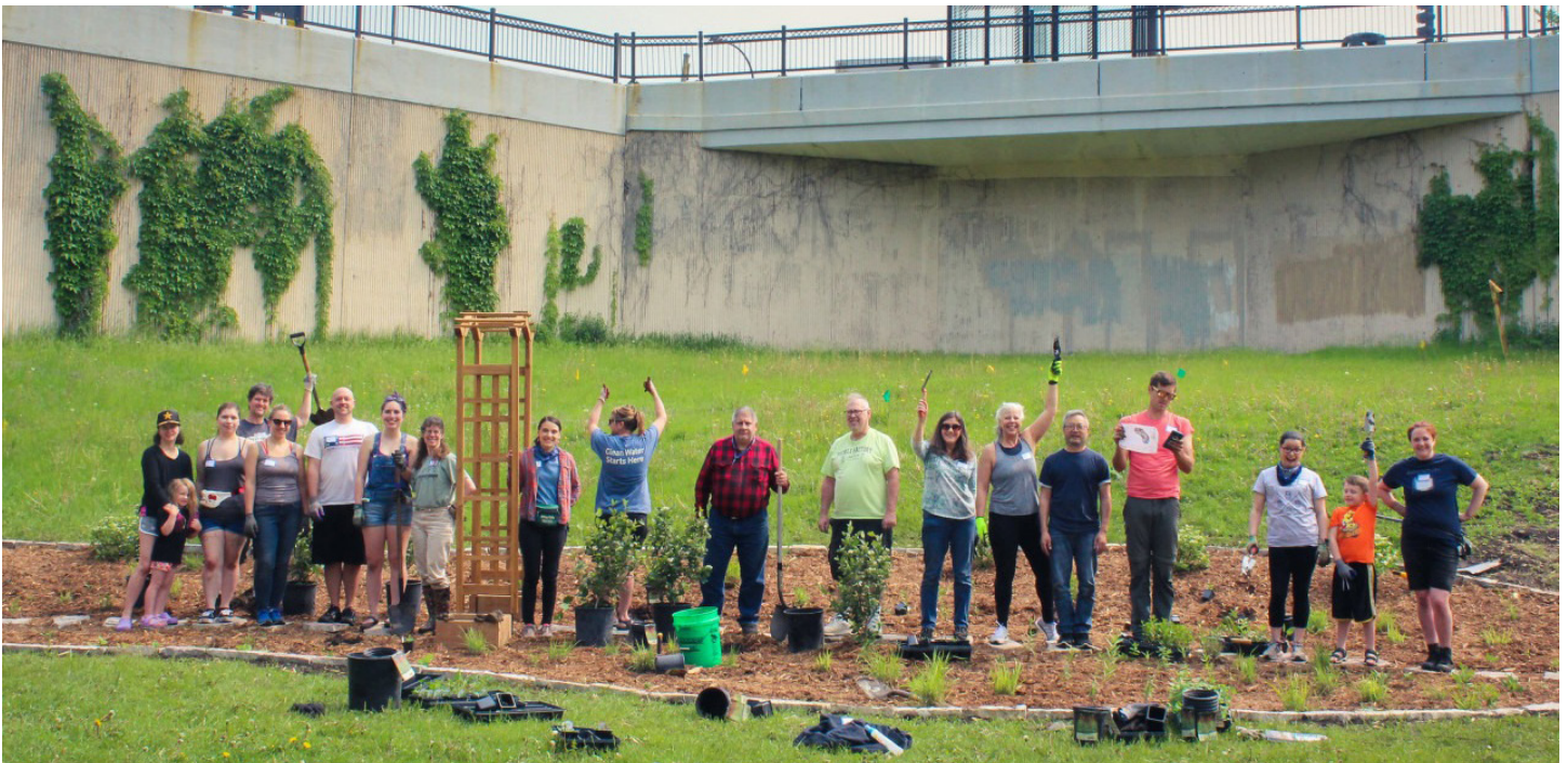
Installation of rain garden at Community Commons Park, Minneapolis, as part of MWS Christina Perfetti's capstone project. Photo credit: Mississippi Watershed Management Organization.
